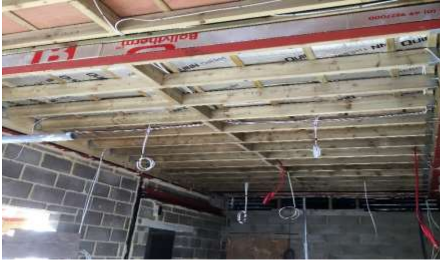
Photo on left shows construction of new office and reception area at first fix stage.
