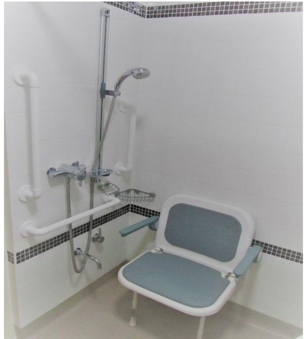
Level access shower room comprising thermostatically controlled electric shower, DDA compliant seat and non-slip safety flooring
