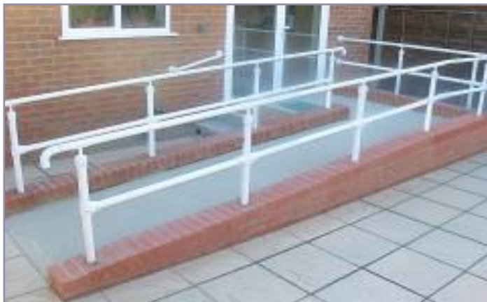
Wheel chair users ramp with powder coated part M compliant handrail system.
