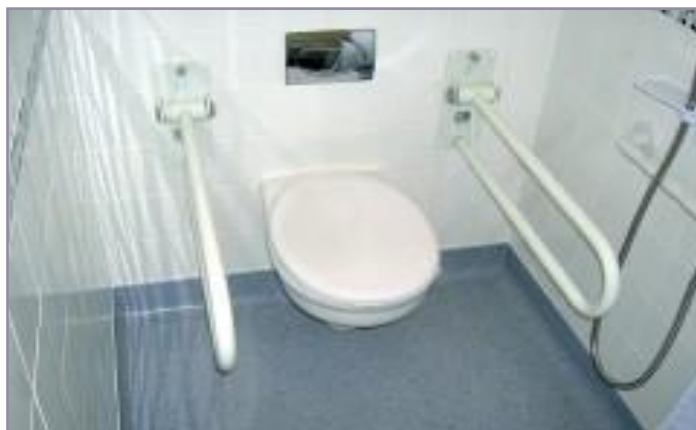
Level access shower room comprising wall hung WC pan, drop down hand rails and non-slip safety flooring
